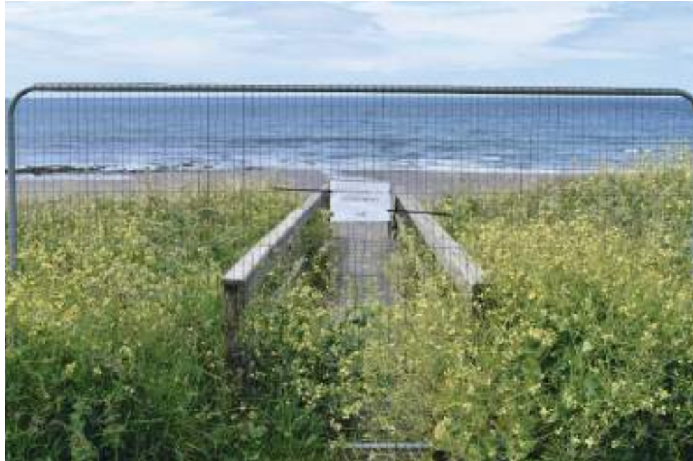
Image 01 - Boardwalk bridge in need of repair
