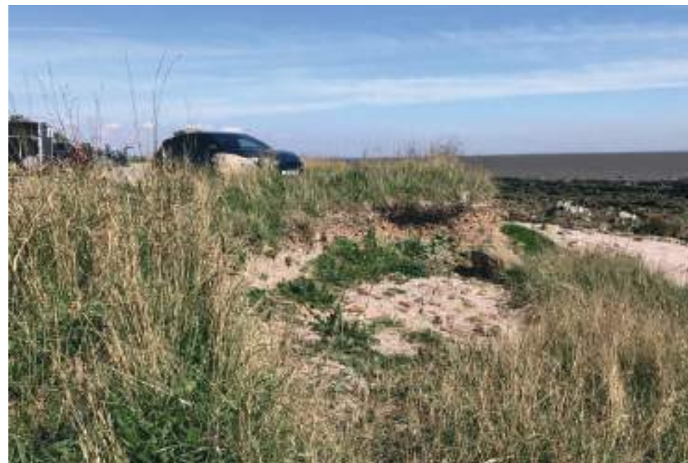
Image 05 - Erosion/damage of adjacent landscape
